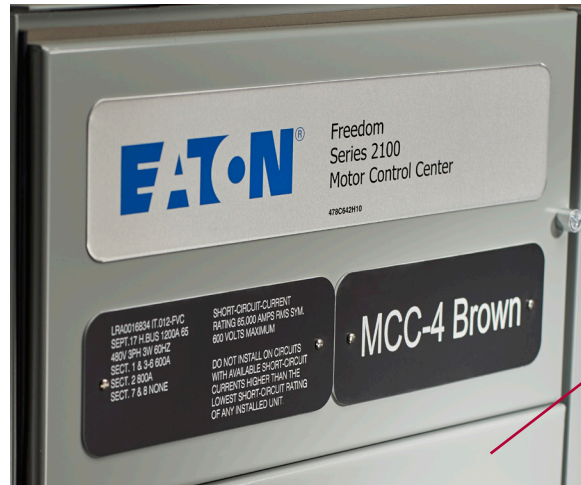
Manufacturer's nameplate with MCC SCCR marking: 65,000 A rms sym at 600V max.
