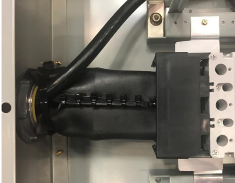
Lineside barrier provides protection from incidental contact.
