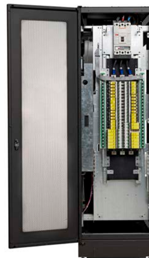
Figure 8.1.8.2.c Eaton RPP with QSCP chassis.
