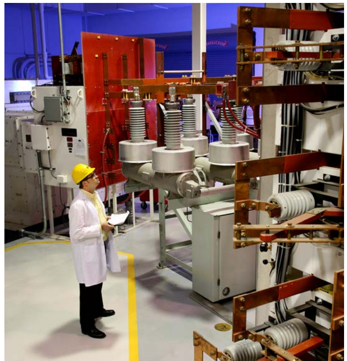
The Eaton Bussmann Division’s Paul P. Gubany Center for High Power Technology is the electrical industry’s most comprehensive facility for testing and certifying device and equipment SCCRs. Capable of performing electrical tests up to 600 V three-phase, 300 kA fault current for meeting ANCE, ANSI, CE, CSA, ETL, IEC and UL testing requirements.
