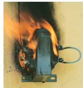
Figure 3.1.4.2.b Fires can result if the correct OCPD amp rating is not applied.
