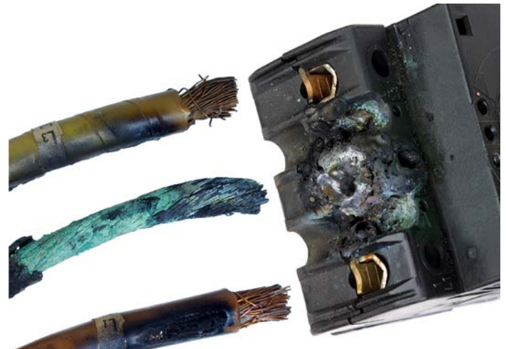
Figure 7.7.7.a This disconnect’s middle, lineside conductor became loose and created an excessive thermal condition that damaged the terminal, along with the middle and the adjacent conductors.
